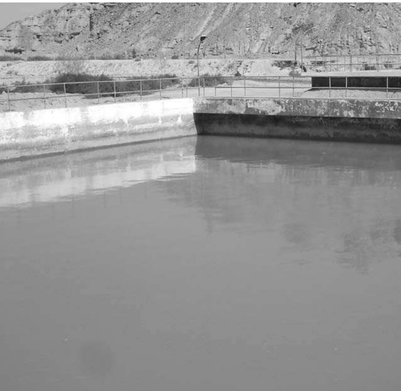
Sand filter bed for supplying drinking water from Ankra Kaur Dam reservoir to Gwadar Town and surrounding areas
